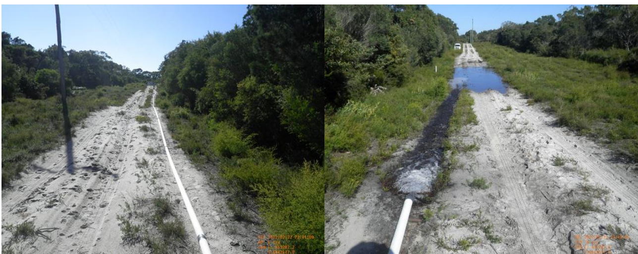
Photo 3 on the left shows the discharge pipeline and Photo 4 on the right shows the ponded discharge.
